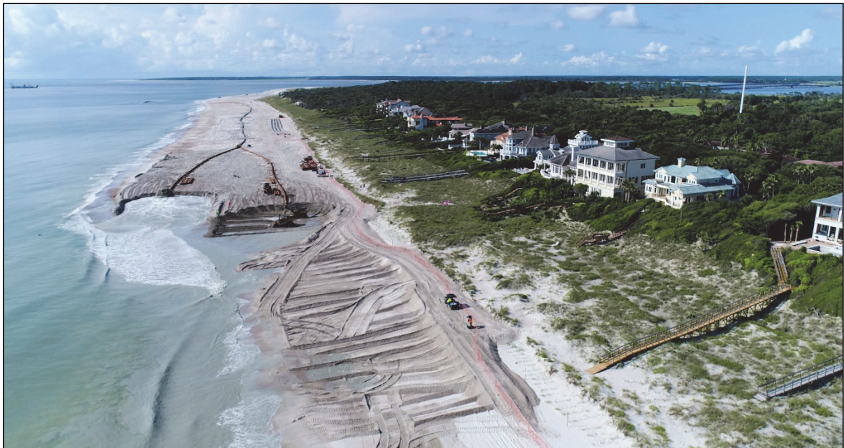
Photograph 1.1: Southward view of the beach fill construction progress at The Residence on 11 Aug, 2021 near Station 65+00 (R-72).
